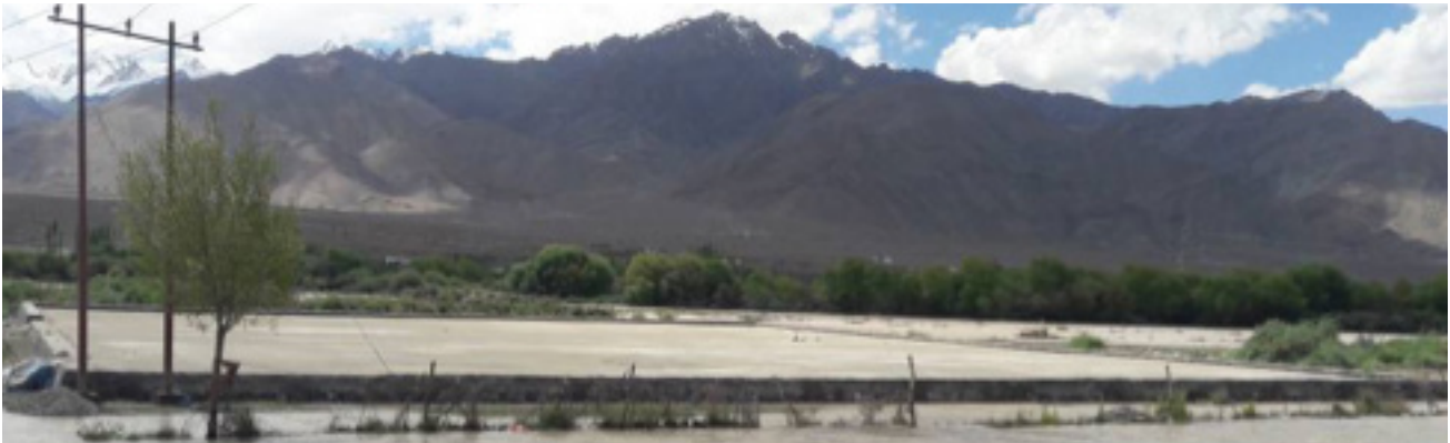
Land development, access bridge and parking area development works at Choglamsar, Cluster Spituk, Leh
