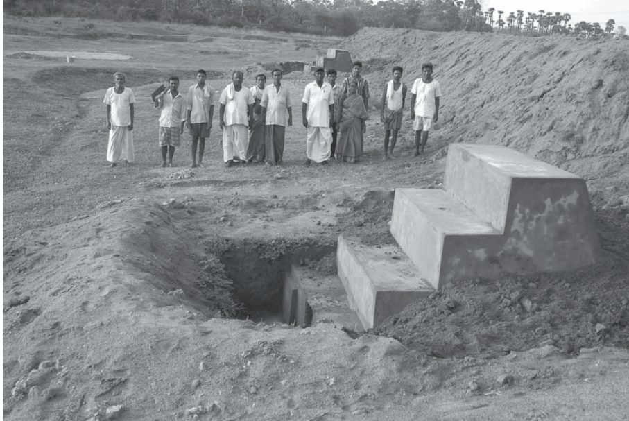
Sarpanch and villagers showing constructed Sluice of MI tank in Malluru village of Warangal district
